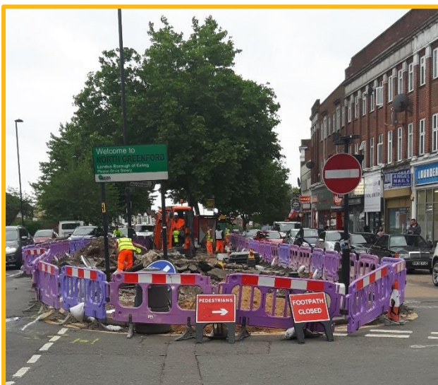
Looking south from Sudbury Hill Underground Station: Work to improve the footway between Greenford road and the service road.
